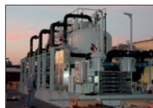
Produced water unit with BOLLFILTER Automatic type 6.18, grade of filtration 50 micron
